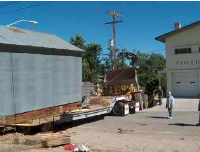
The cab of the flat-bed is turned sideways and the powder magazine is dragged aboard with a loader.
